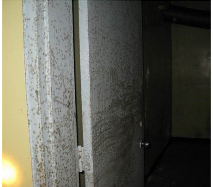
Mold growth in poorly ventilated space
