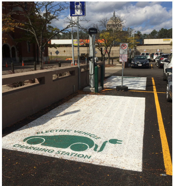
Electric Car Charging Station
