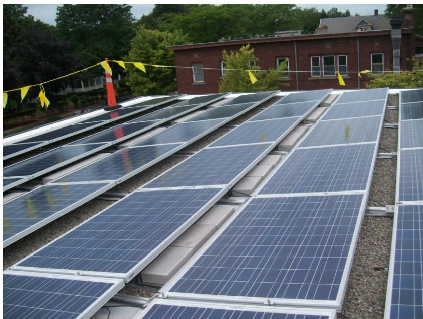
Photovoltaic cells on Arnett Library.
