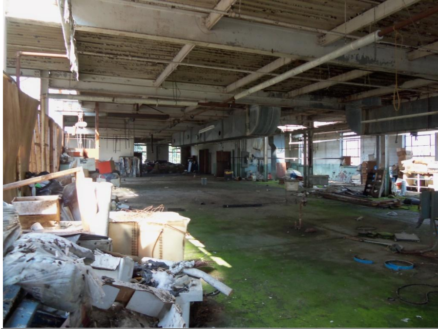
View of second floor, looking west. Roof deck spans left-to-right (north-south) over 8" deep roof channels spaced at 8" o.c.. Channels span east-west. Steel beam spans left-to-right (north-south)
