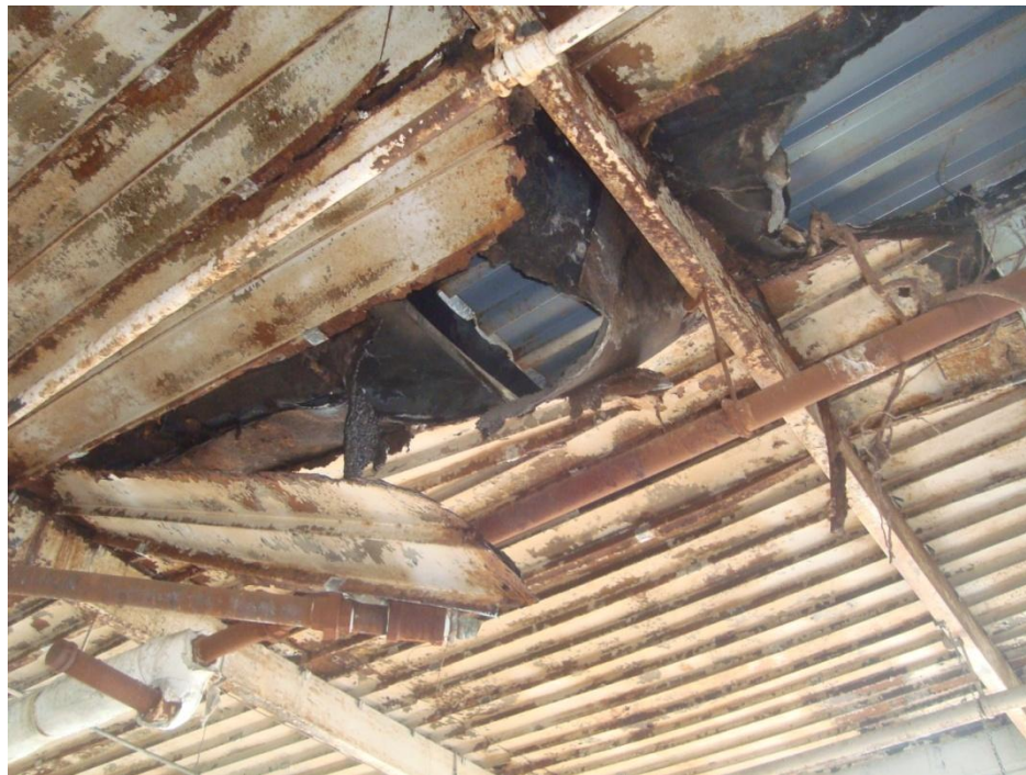
View of collapsed area of roof deck
